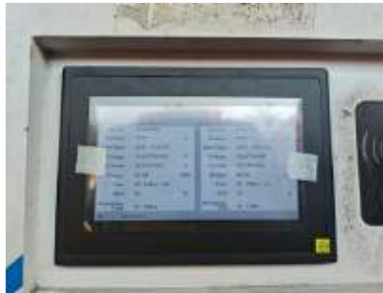
Parameters Displayed on the EV Charger Screen
