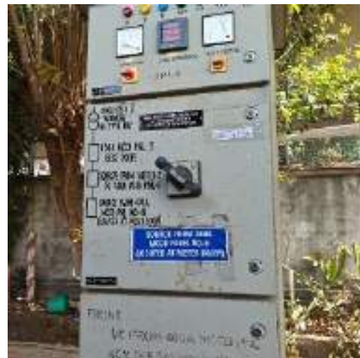
No danger warning board
