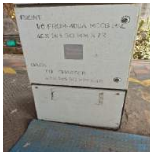
Protective rubber mats in front of DB
