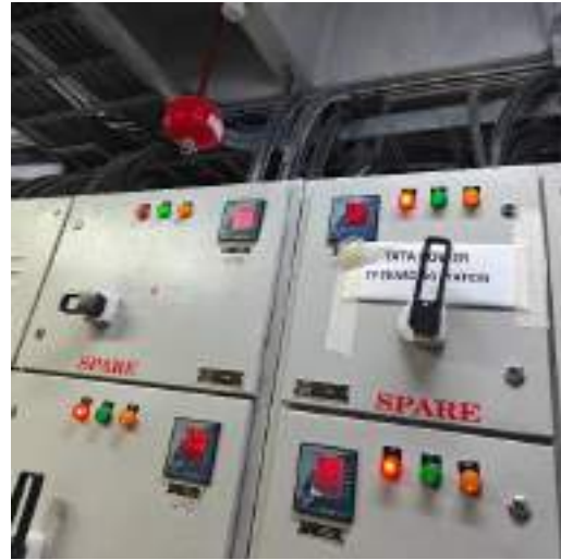
Nonfunctional smoke detector
