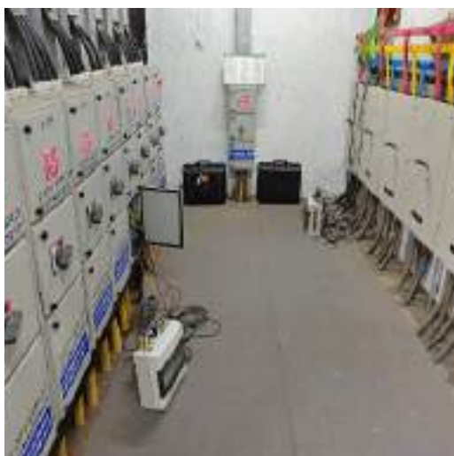
Protective rubber mats in front of panel
