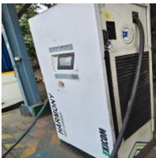
Protective rubber mats in front of Charger
