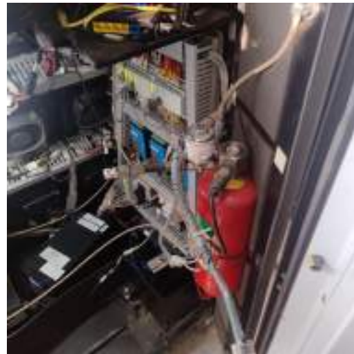
Automatic fire suppression system
